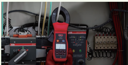
Measurement of AC Current in Distribution Cabinets
