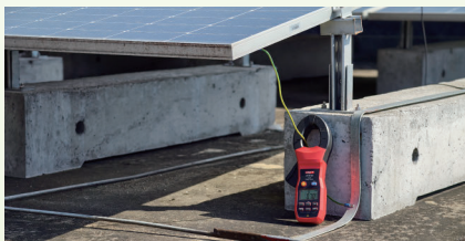
Measurement of Ground Resistance of solar Panels
