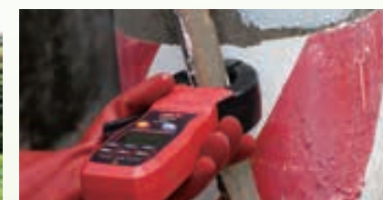
Measurement of Transformer Ground Resistance
