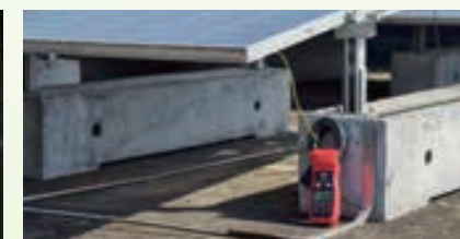
Measurement of Ground Resistance of solar Panels
