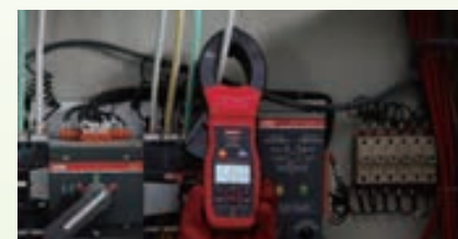
Measurement of AC Current in Distribution Cabinets
