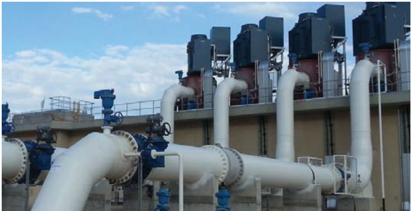
Water pump station at Mekorot Israel
